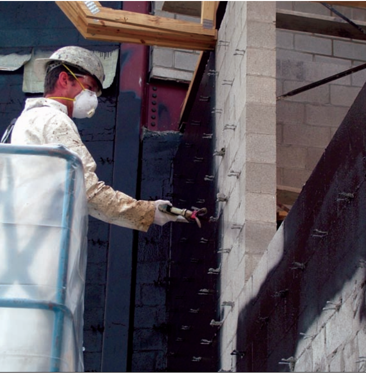
Details at corners, changes in plane, and brick ties are included during the field application process. Cold-applied liquid barriers can make the process considerably more efficient.
