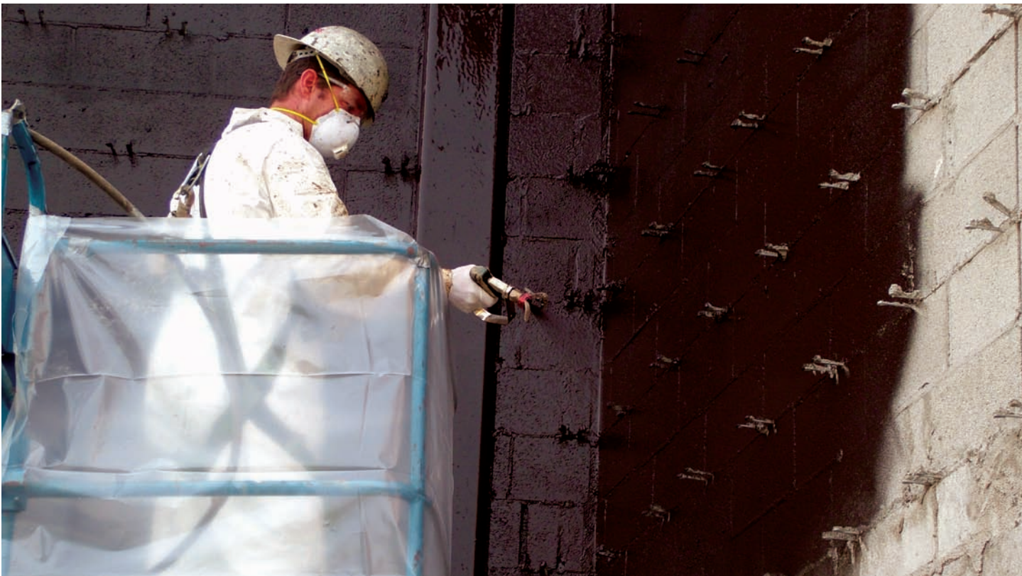
Spraying on a liquid air- and vapour-barrier can achieve rapid application rates over dissimilar substrates.
