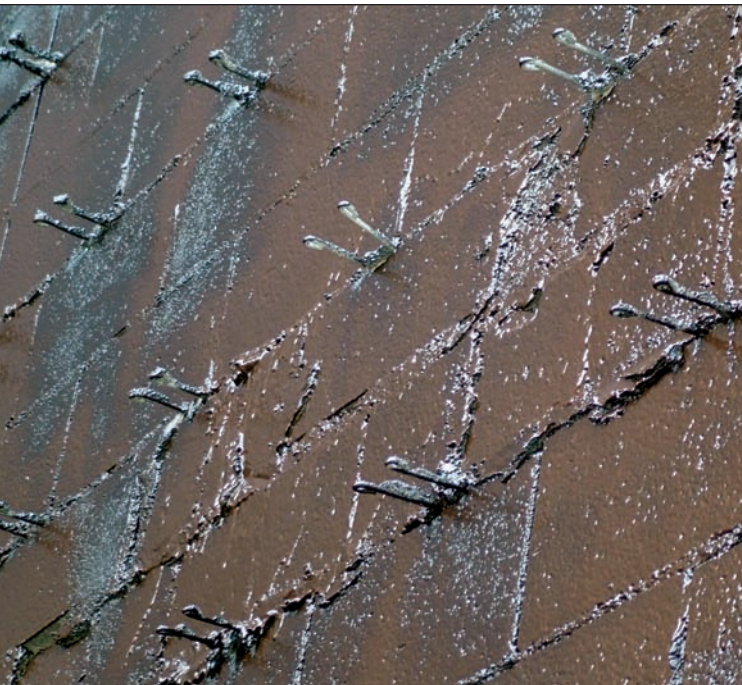
A well-bonded, monolithic membrane can easily be achieved on uneven surfaces. Above, a good seal was accomplished around the brick ties during the initial application process.
