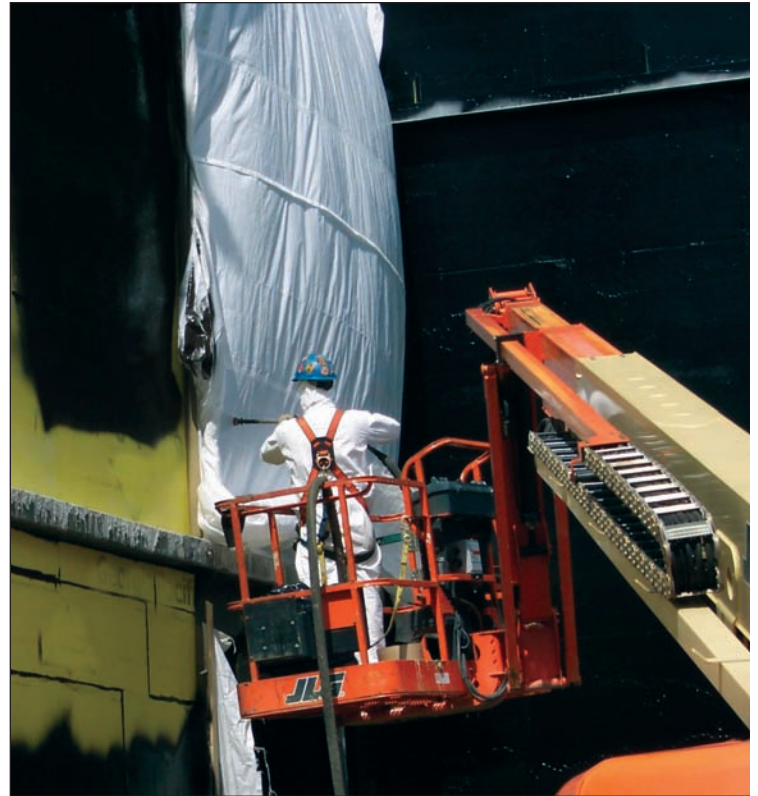
Cold-applied, liquid air- and vapour-barriers adhere well to exterior-grade sheathing boards as seen above.
